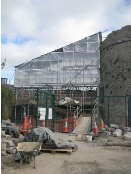
The covered scaffolding viewed from the west. The size and scale of the building allowed for a ramped access rather than the traditional method of ladder access. This was a more efficient way of carrying stone and wheelbarrows of lime mortar.
