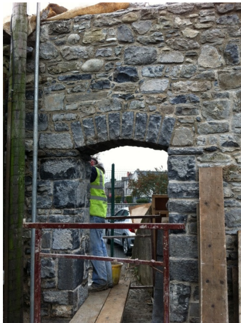
The completed section of north curtain wall, with new arch built to match the arch of the tower. The Irish oak gate has been manufactured and will be fitted when all scaffolding has been removed
