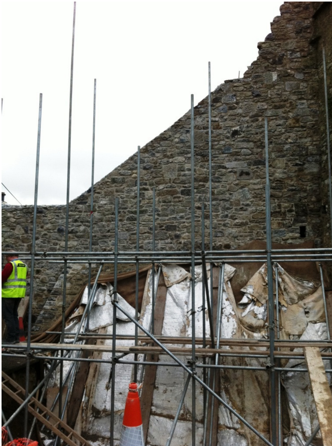
The completed west wall, with the protection still on the base batter. Note that the top section was the only extant section of the wall.
