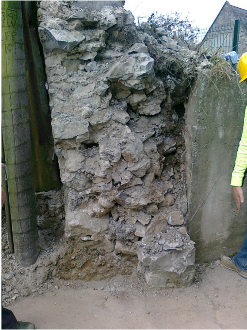
The section of north curtain wall was in imminent danger of collapse.
