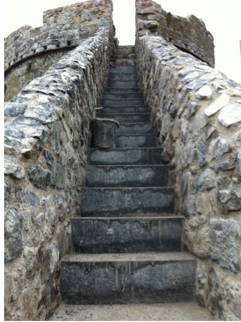
The completed steps. The new steps marry into existing steps, with a steep rake at the upper level.
