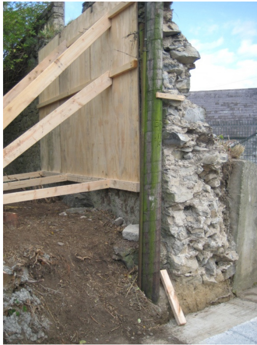
The wall was surveyed, carefully taken down. A new foundation was poured after the site was excavated by an archaeologist and the remainder of the wall has been supported with a temporary buttress.
