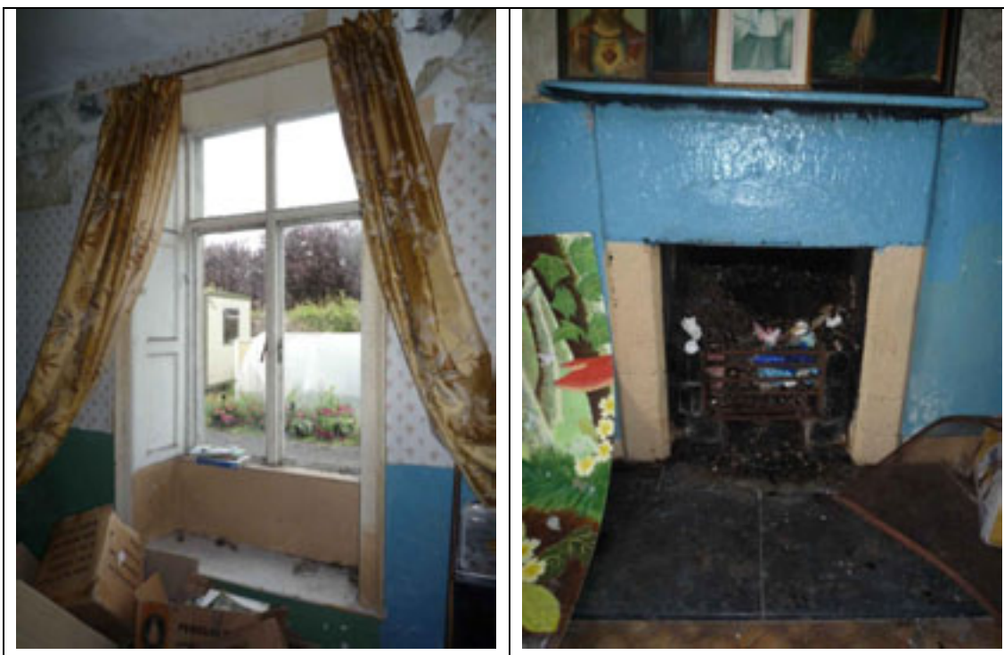
Fig.49: Window opening showing timber panelled shutters. Fig.50: Fireplace to east wall having painted stone surround, timber mantel shelf and modern limestone hearth.
