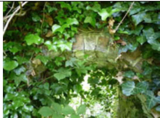
Fig.34: Archway giving access to the heavily overgrown former sanitary block located to the southeast of the site.
