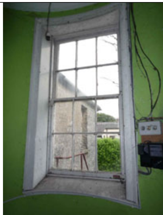
Fig.166: Window opening in the east wall with early timber sash window. Note the architrave follows the curve of the room.
