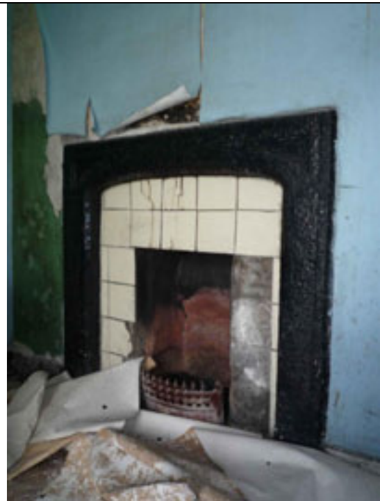
Fig.206: Over-painted stone fireplace with modern tiled insert.
