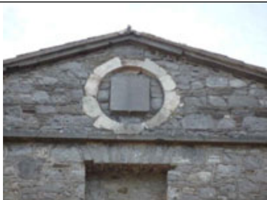
Fig.11: Plaque to central pedimented breakfront of principle/west elevation set within circular recessed panel.
