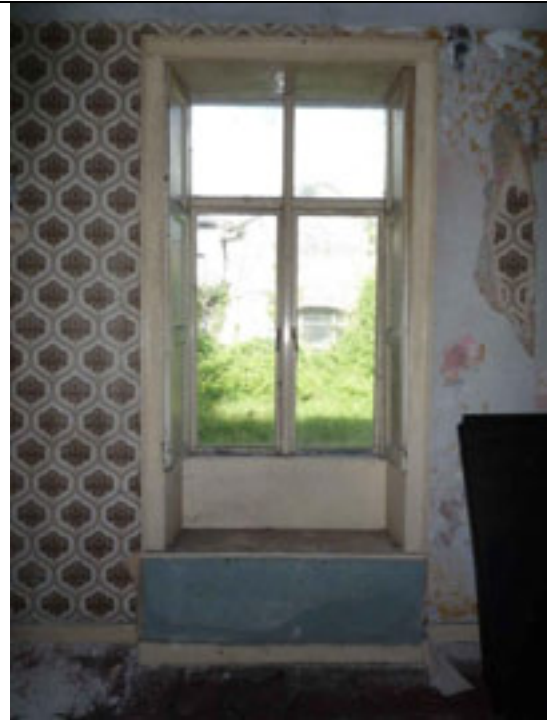
Fig.112: Early timber window joinery. Note the architrave rests on a projecting window apron.
