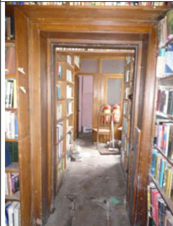
Fig.87: Door opening to south wall giving access to G16. Note the door is missing.
