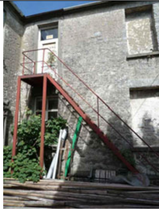
Fig.22: Emergency fire exit stair and door (former window ope) to northern wing.
