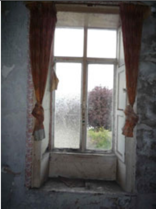
Fig.137: Window opening with surviving timber joinery. Note the shutter to the left is missing.
