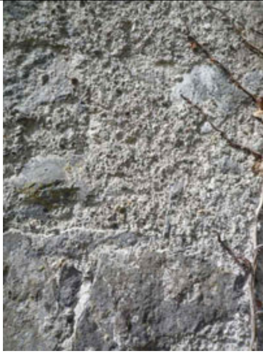
Fig.9: Traces of surviving lime based harling to east elevation with exposed aggregate of varying size.
