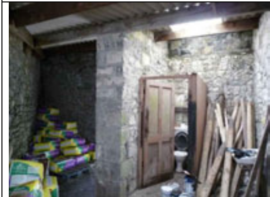
Fig.33: Interior of the former sanitary block to the northeast of the site. Note the limestone wall subdividing the space.
