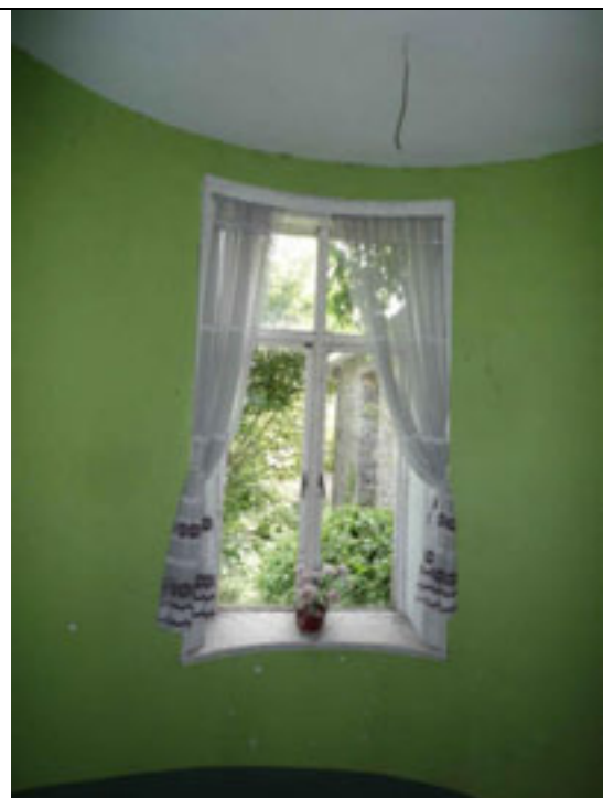
Fig.190: Window opening in the east wall. Note the architrave follows the curve of the room.
