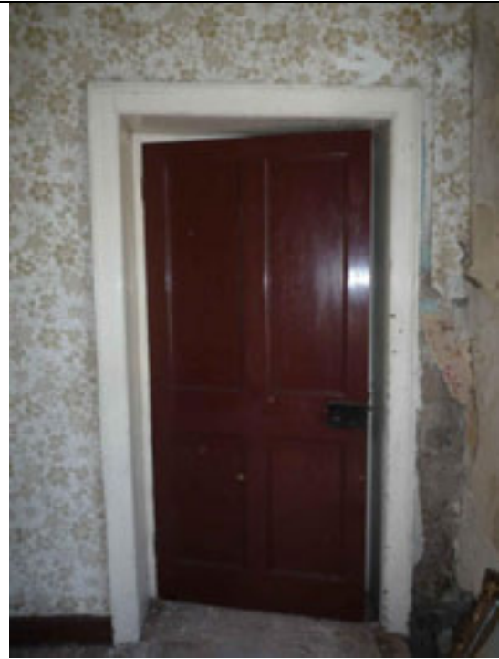
Fig.178: Timber panelled door in the south wall giving access to room F16.
